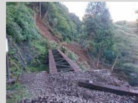
Track bed washout
