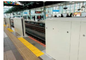
Platform doors on the down-train platforms (platform 1 and 2) Noborito Station
